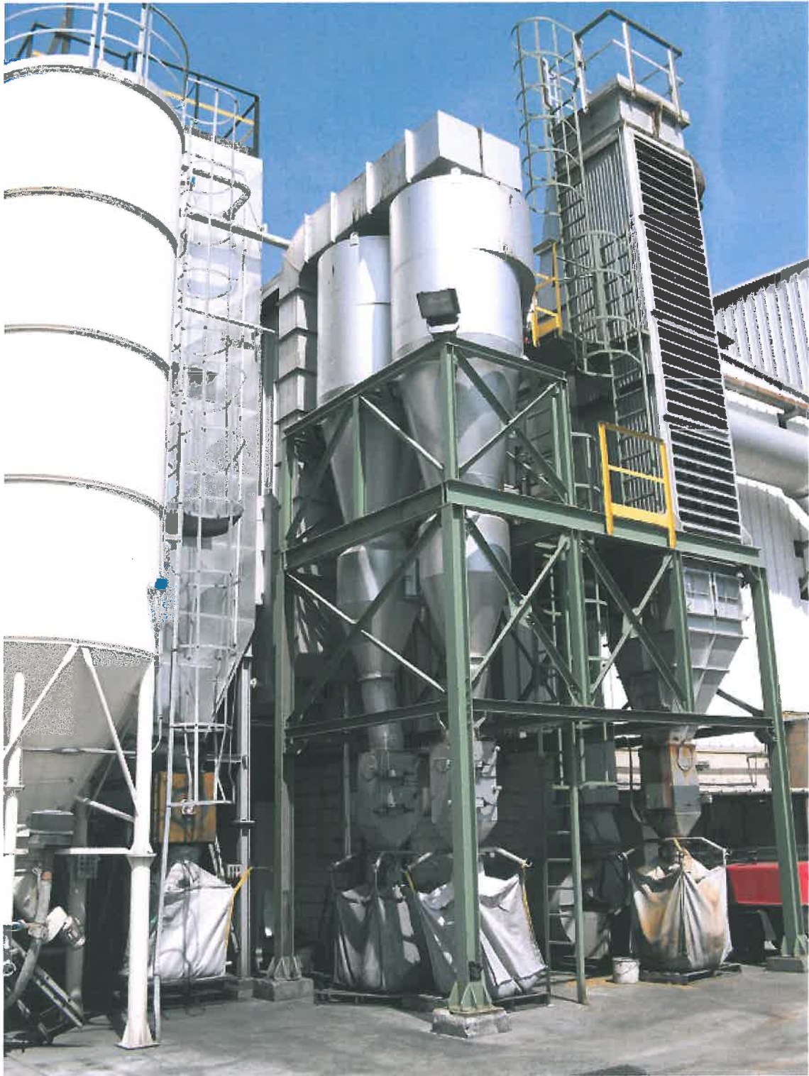
POST COMBUSTION CAPTURE
